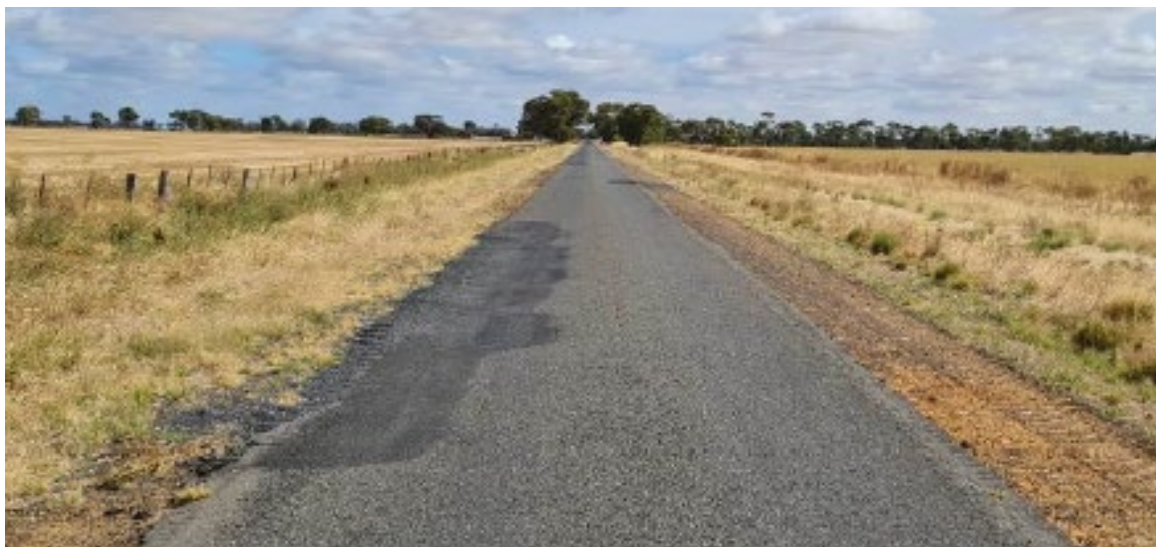
Figure 4.0 – Typical condition of Lorquon Road following damage in 2022
