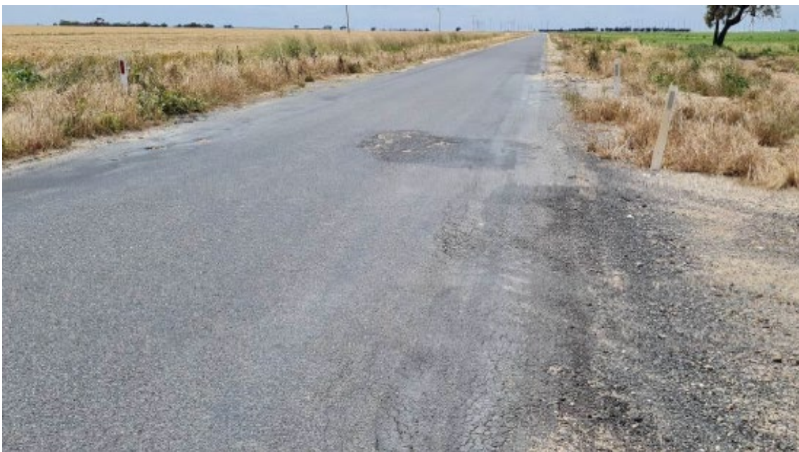
Figure 2.0 – Typical condition of Dimboola-Minyip Road taken following damage in 2022.
