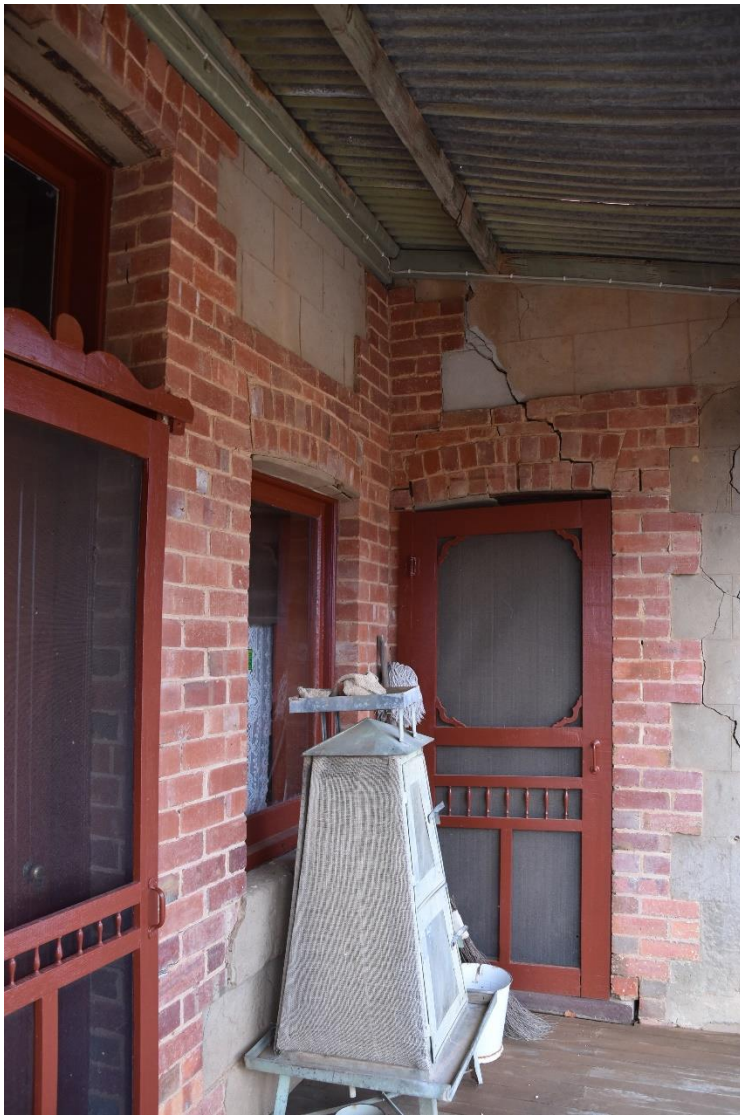
Figure 1: The western verandah showing subsidence and cracking near the laundry door.
