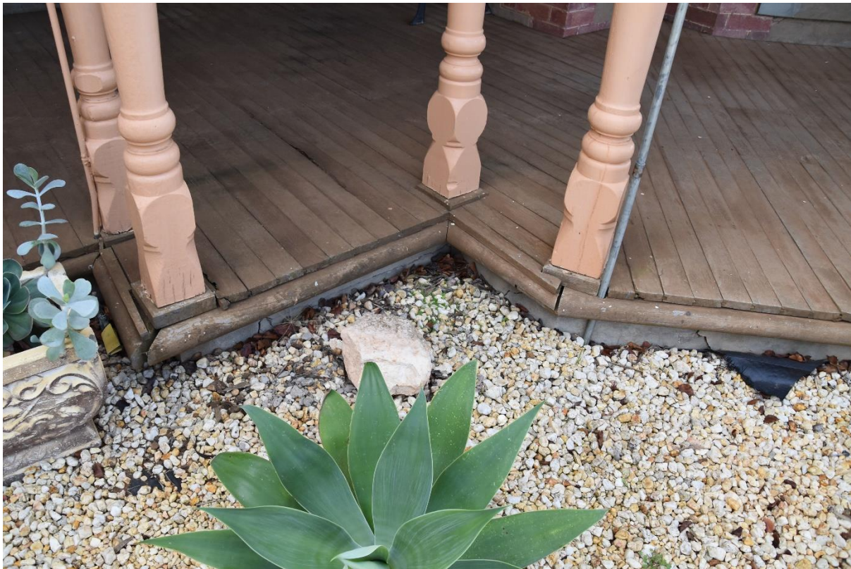
Figure 3: Overly high ground level on the southern side.
