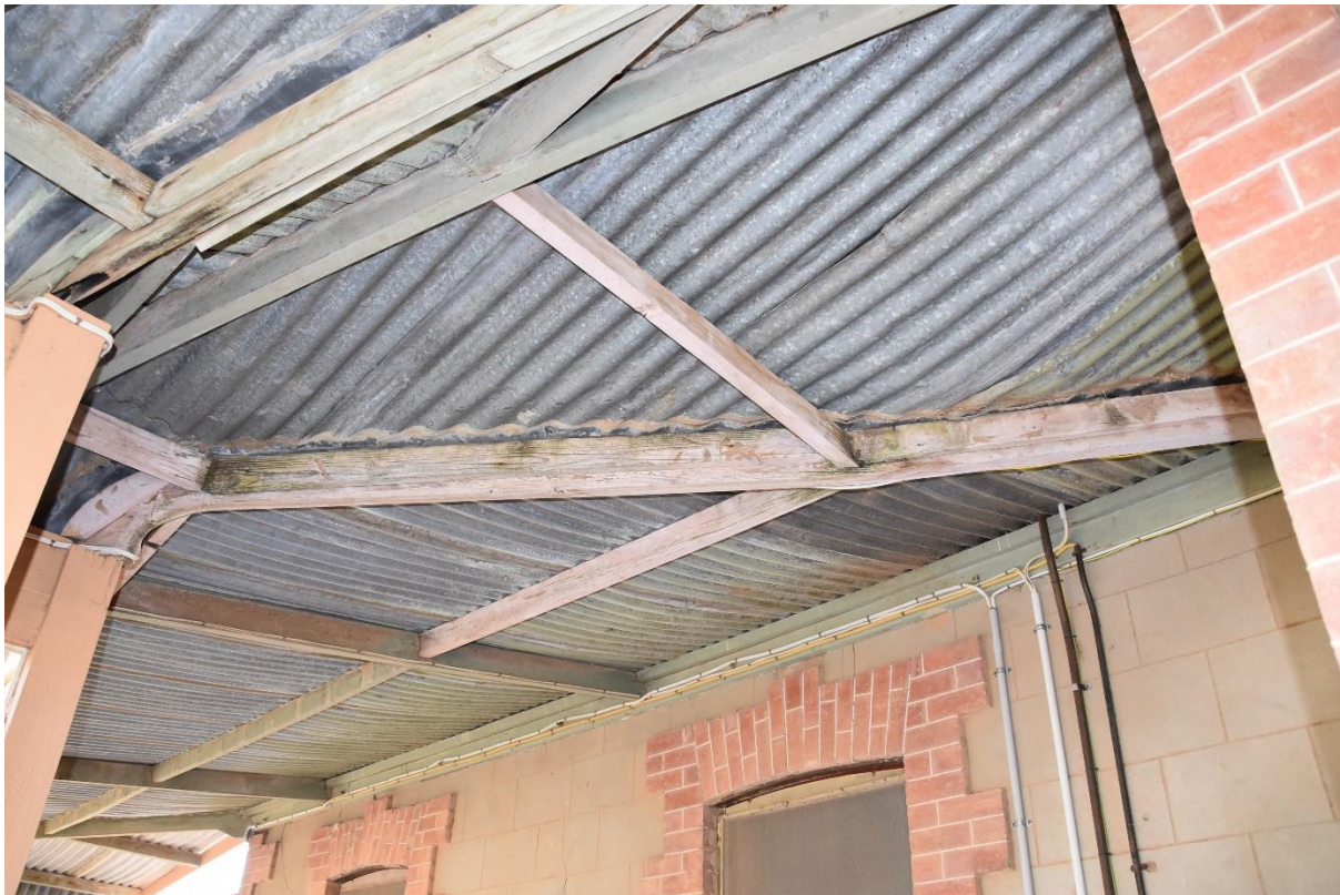
Figure 2: Structural issues in the verandah near the dining room.
