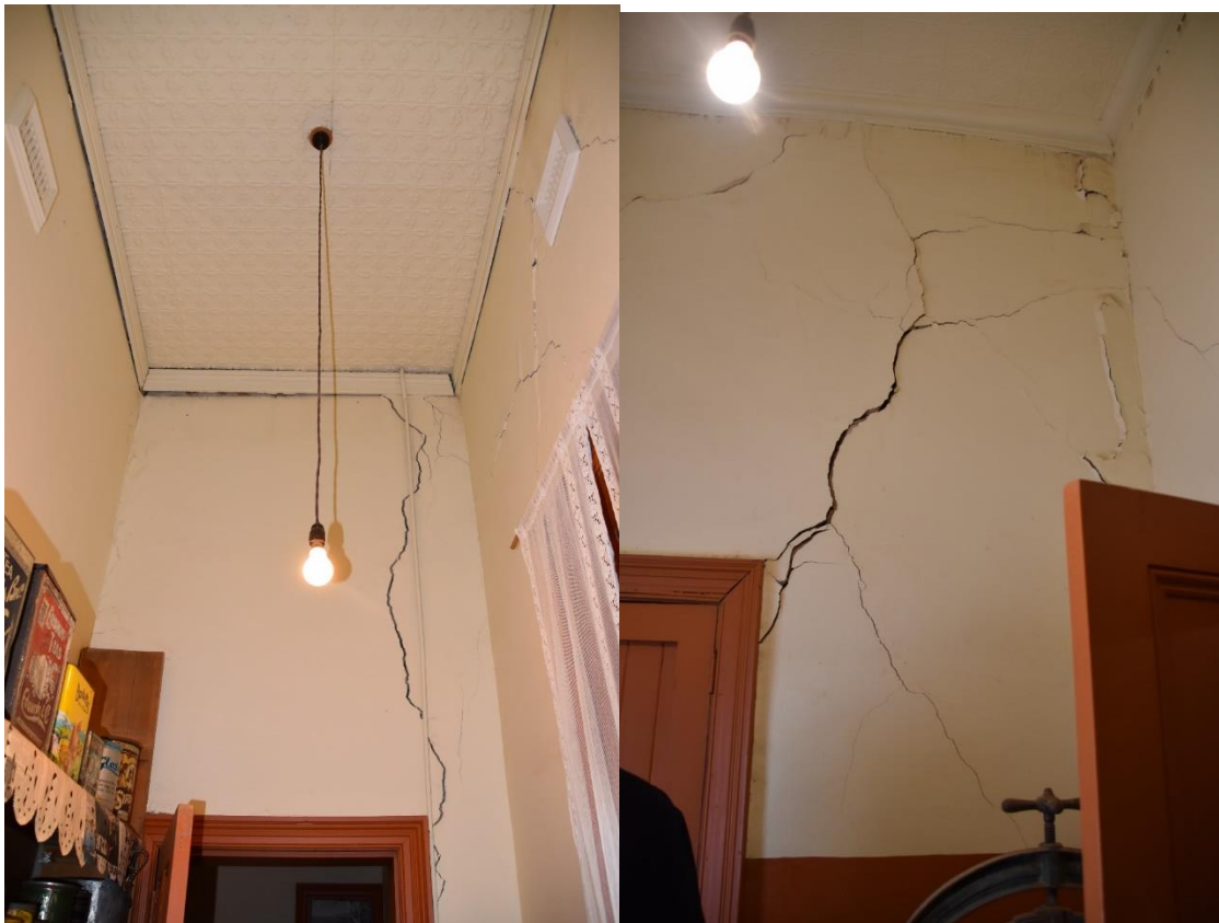
Figure 4: Serious issues in pantry and laundry.
